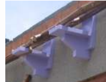
The wooden joint at the junction beam & the wall
